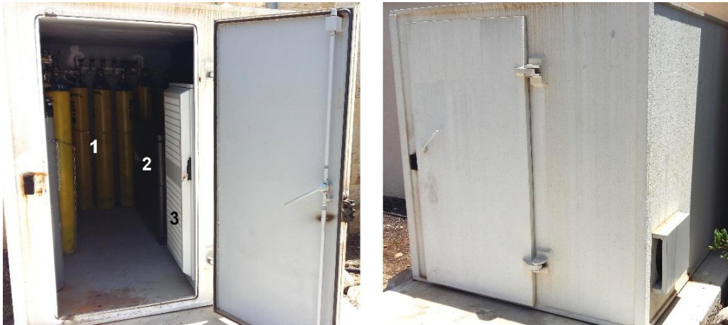
Fig. 6. The FCs with balloons, inverter, and batteries enclosed in special steel box of 2m x 3m x 2m: 1 – set of standard hydrogen balloons 150 atm; 2 – electrochemical cell; 3 – inverter and batteries.
